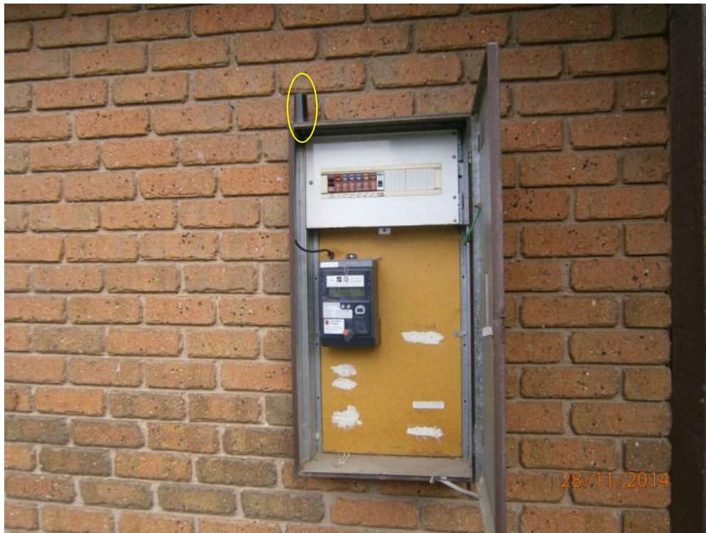
Photo B.3 Mesh – Individual Meter Site – External Antenna
