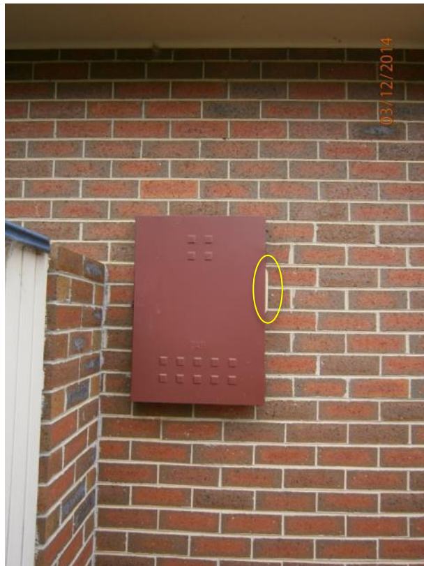
Photo B4 WiMax – Individual Meter Site – Externally Mounted Antenna
