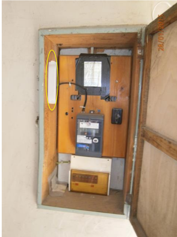
Photo B.5 WiMax – Individual Meter Site – Internally Mounted Antenna
