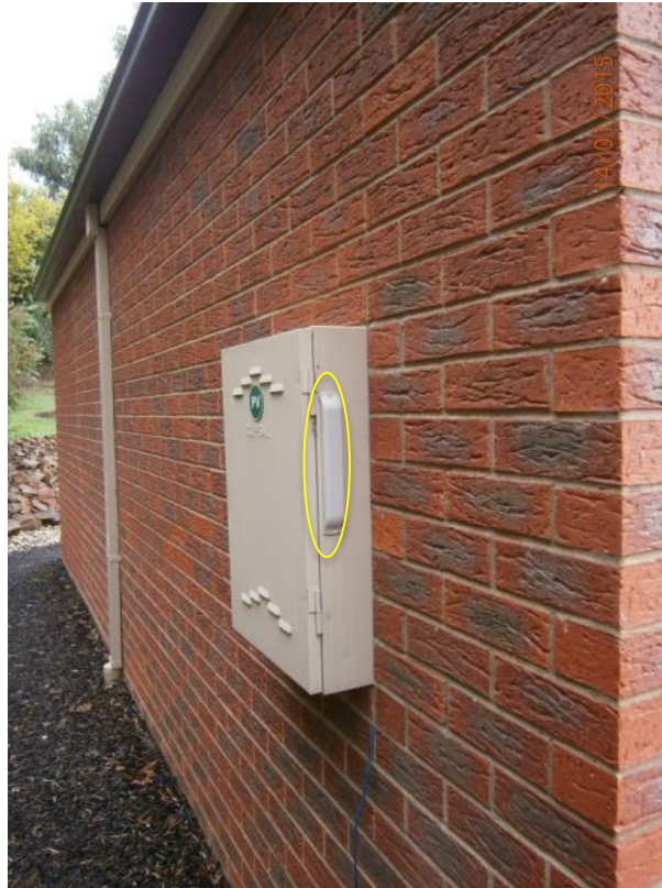
Photo B.7 3G – Individual Meter Site – Externally Mounted Antenna
