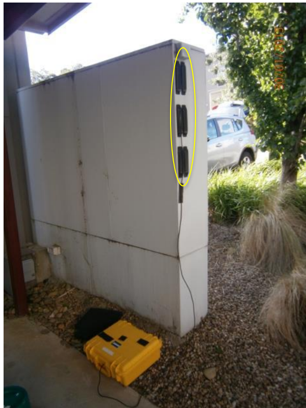
Photo B.6 WiMax – Group Meter Site - External Mounted Antennas
