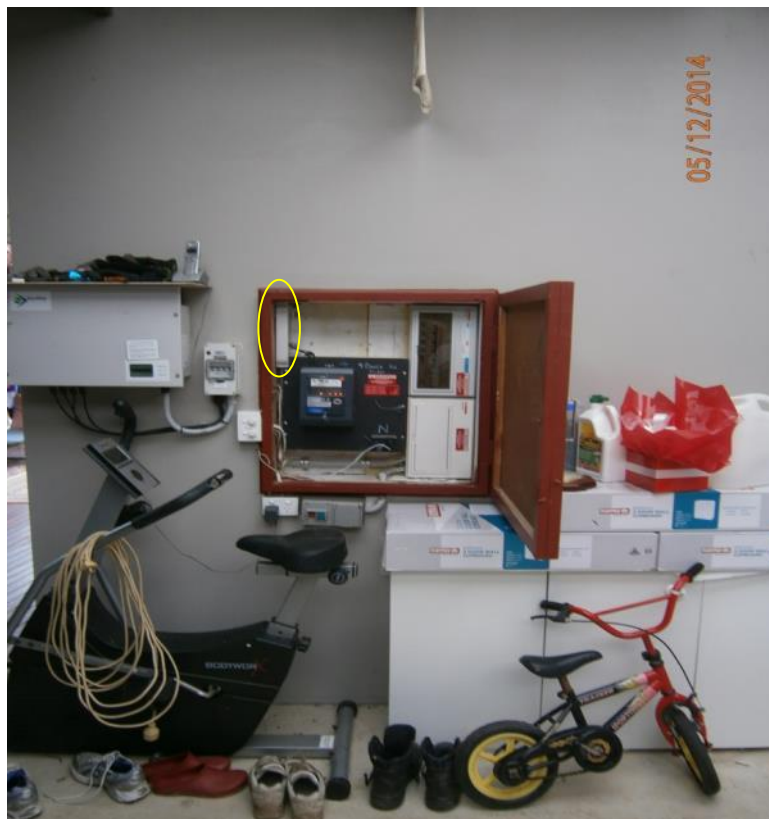
Photo B.8 3G – Individual Meter Site – Internally Mounted Antenna
