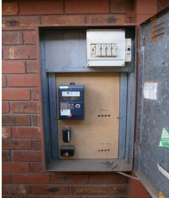
Photo B.1 Mesh – Individual Meter Site – Internal Antenna
